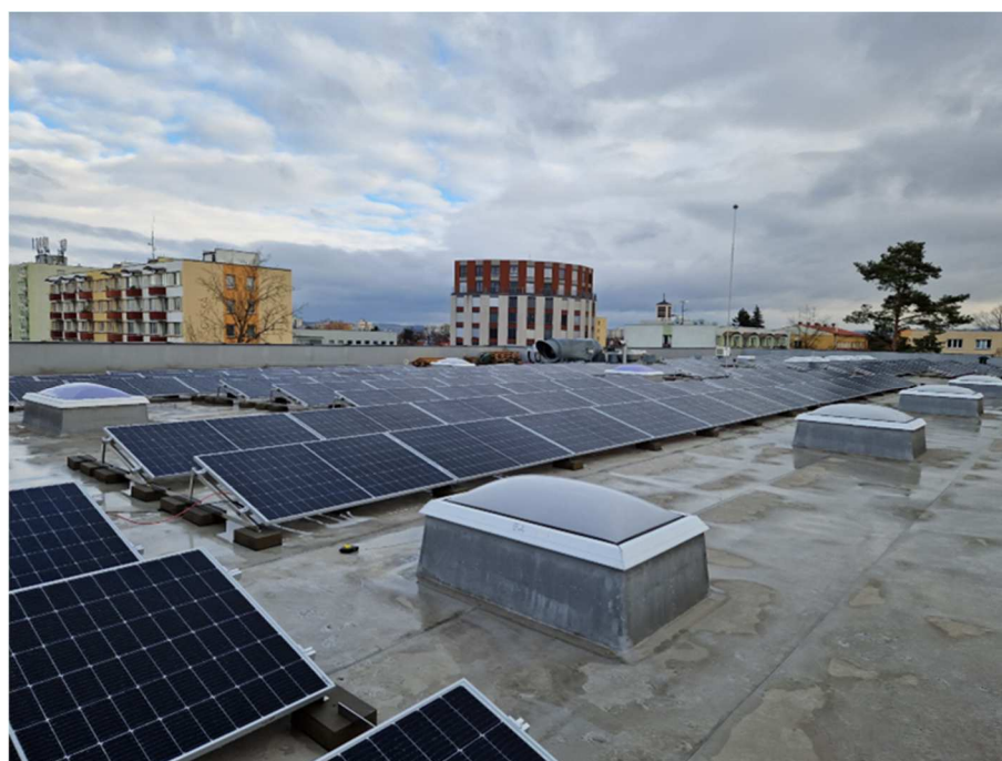
Installed PV, USB Academic Library building. Photo: USB Project Office.
