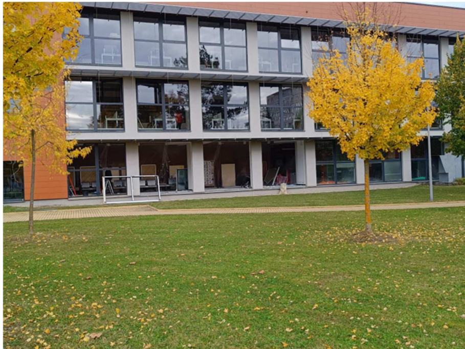
Ongoing window replacement work, USB Academic Library building. Photo: USB Project Office.
